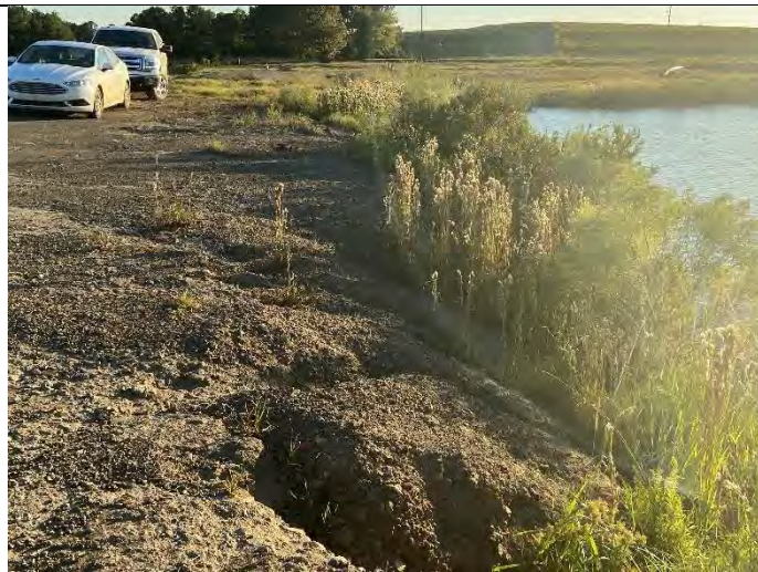
Photograph 3: Close-up view of upstream edge of upstream slope overbuild. Note erosion gullies. Since gullies have formed in the overbuild material, they are not considered problematic.
