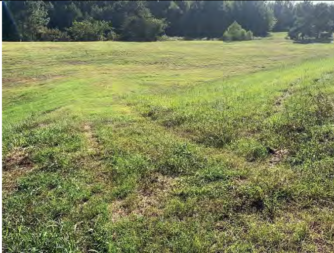
Photograph 17: View of access ramp leading up to crest at southwest corner of pond.
