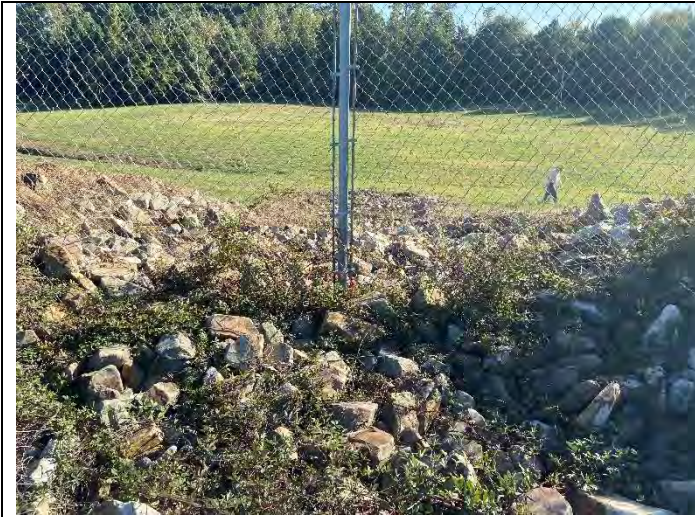
Photograph 10: View of emergency spillway outlet channel, looking downstream. Note crest fence partially blocks the spillway weir.
