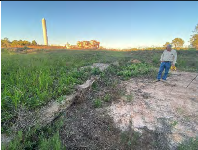
Photograph 11: Close-up view of primary emergency spillway overflow weir. Note undermining damage on upstream and downstream faces, and overall irregularity of the weir.
