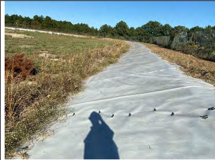
Photograph 4: Typical view of upstream slope and geosynthetic liner. East embankment, looking east.
