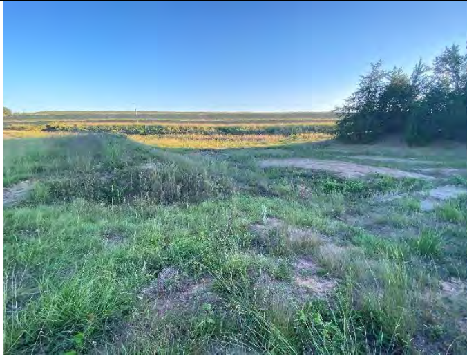
Photograph 10: View of primary emergency spillway, looking downstream, from near the overflow weir location.
