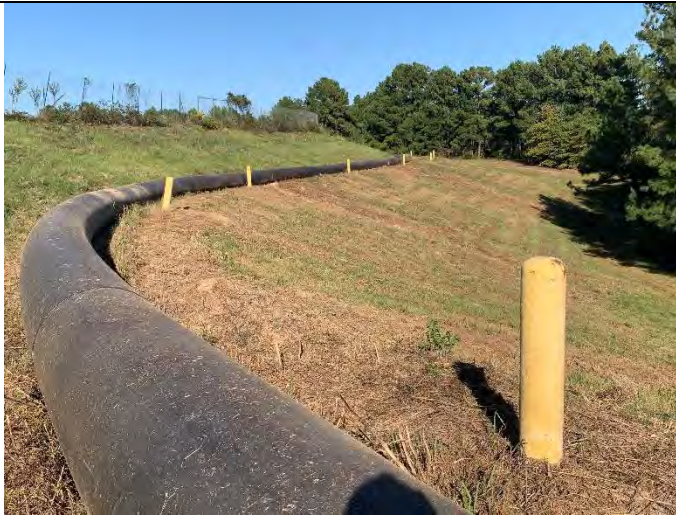
Photograph 16: Typical view of downstream slope and conveyance piping, along east embankment looking east. Note slope is well mowed.
