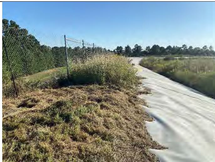
Photograph 6: View of crest where mowing operation had stopped. Beyond this point, the crest of the embankment was overgrown with vegetation and could not be thoroughly inspected. East embankment, near transition to south embankment.
