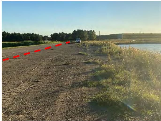
Photograph 2: View along upstream slope, looking right. Superimposed line approximates the original crest upstream shoulder, thus demonstrating the extent of overbuild which has occurred over the original upstream slope.
