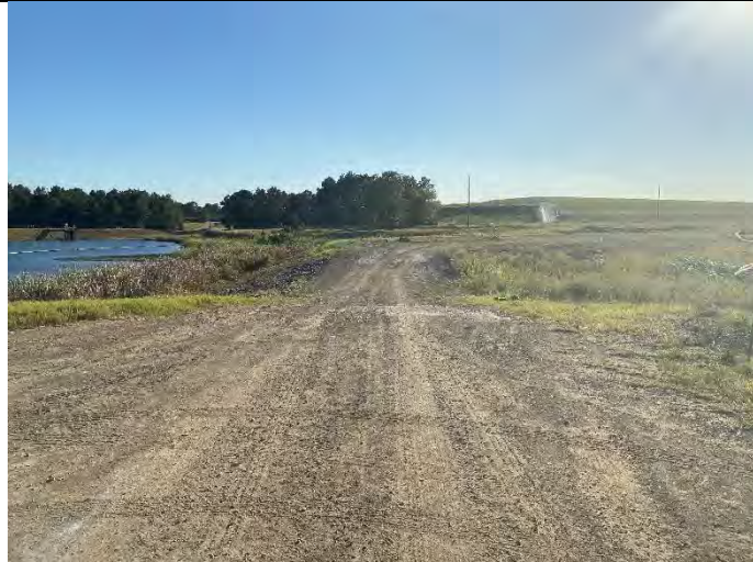
Photograph 8: View along crest, looking right, towards the secondary emergency spillway which had been excavated in the crest/right abutment area. Flow direction is right to left. Clearwater Pond is at left.
