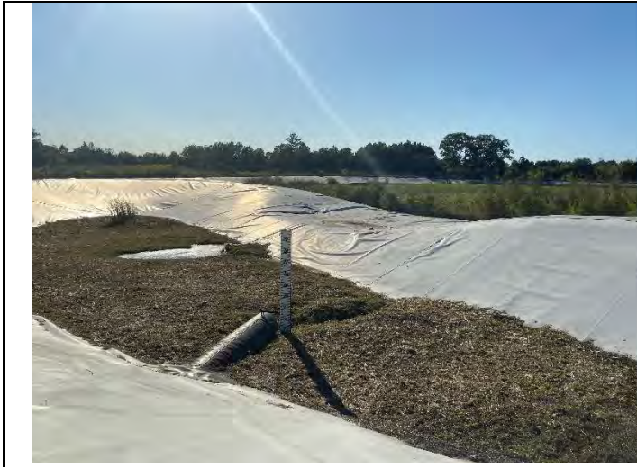
Photograph 7: View of principal spillway outlet pipe and control weir at southeast corner of pond.
