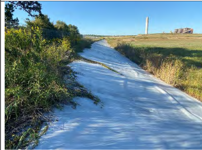
Photograph 11: Typical view of crest and upstream slope on west embankment. Note crest is overgrown with vegetation.
