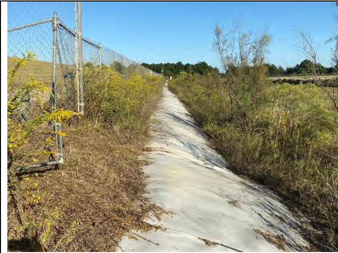
Photograph 13: Typical view of crest and upstream slope on north embankment. Note crest is overgrown with vegetation.
