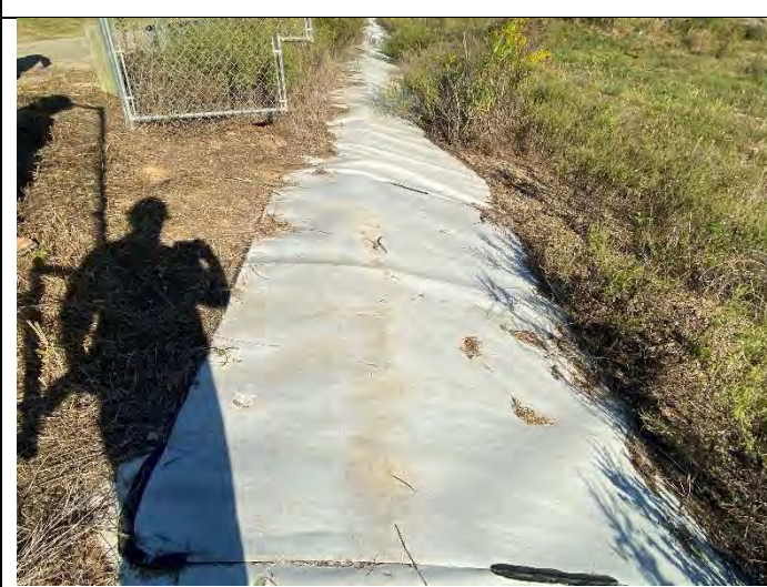
Photograph 14: View of minor abrasion damage of the geosynthetic liner where equipment enter pond through gate at left.
