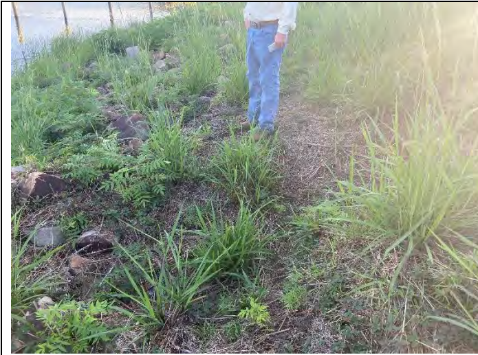
Photograph 7: Example of poor vegetation coverage on downstream slope, near the transition to the rock riprap slope protection. Multiple animal burrows were noted in this area.
